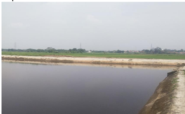
Fig. 6. Damage to Situ Lining
