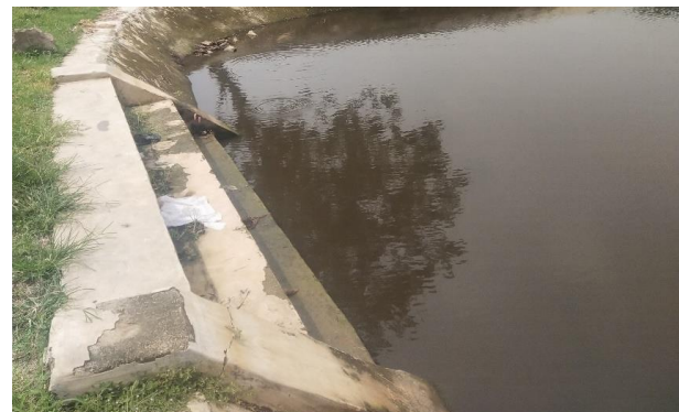
Fig. 7. Damage to Washing Staircase
