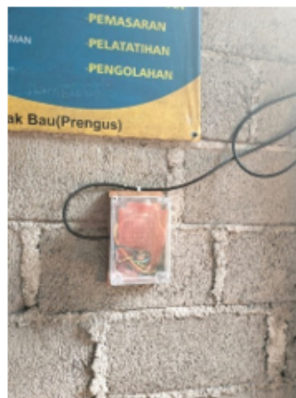
Fig. 9. ESP8266 NodeMCU testing
