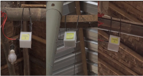
Figure 6. Installed Sensor Node
