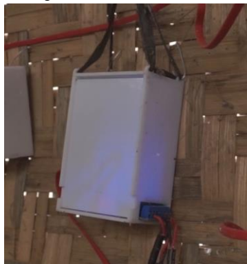
Figure 5. Installed Collector Node
