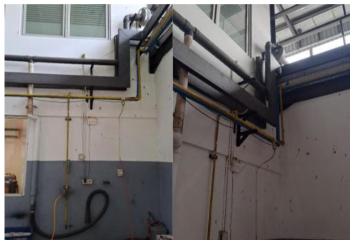
Figure 4. Image After Exhaust System Optimization
