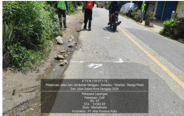
Figure 3. Damage Alligator Cracking
