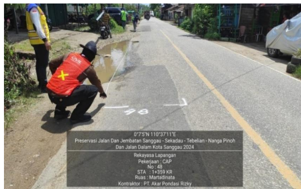
Figure 4. Patch Damage and excavation
