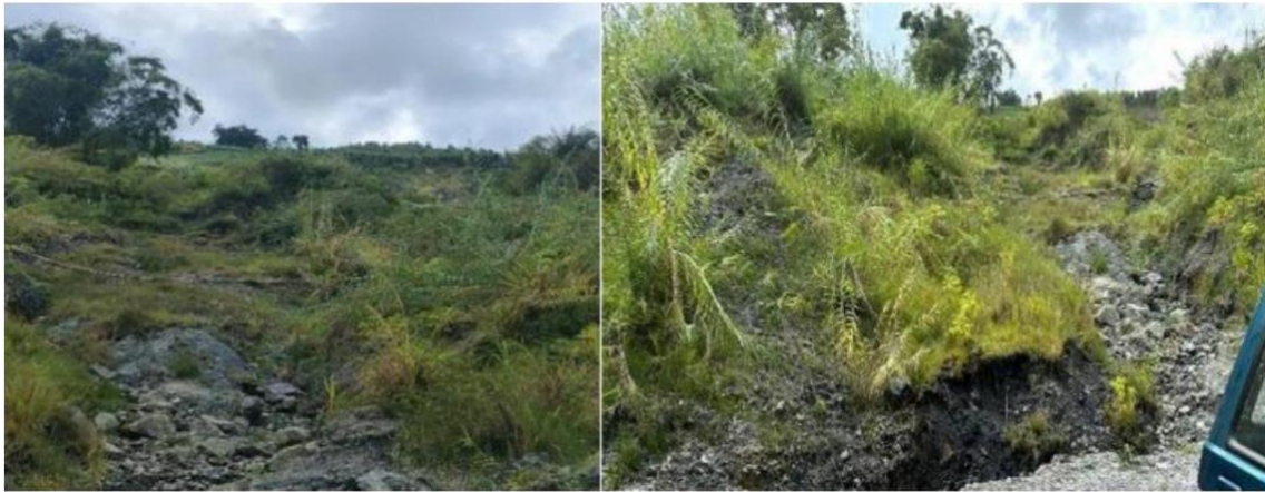
Figure 1. Condition of the slope after the landslide
