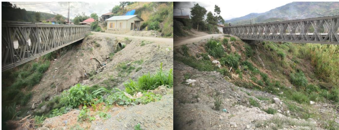
Figure 2. Condition after the slope after the landslide
