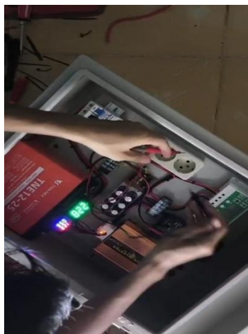
Figure 5. The wind power generator panel box
