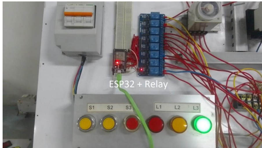
Figure 3. Connecting the ESP32 and 8-channel relay module with contactor, pilot light and timer
