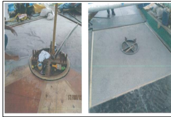
Fig. 8. Installing the first (plywood) and second (white sand) layer dilatation for pierhead
