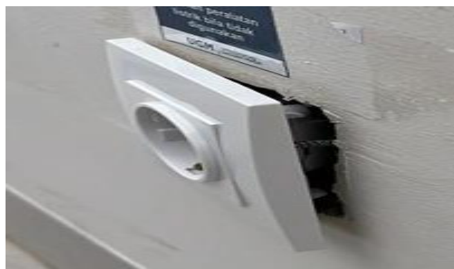
Figure 1. Photo of damage to the utility component of the electrical outlet.
